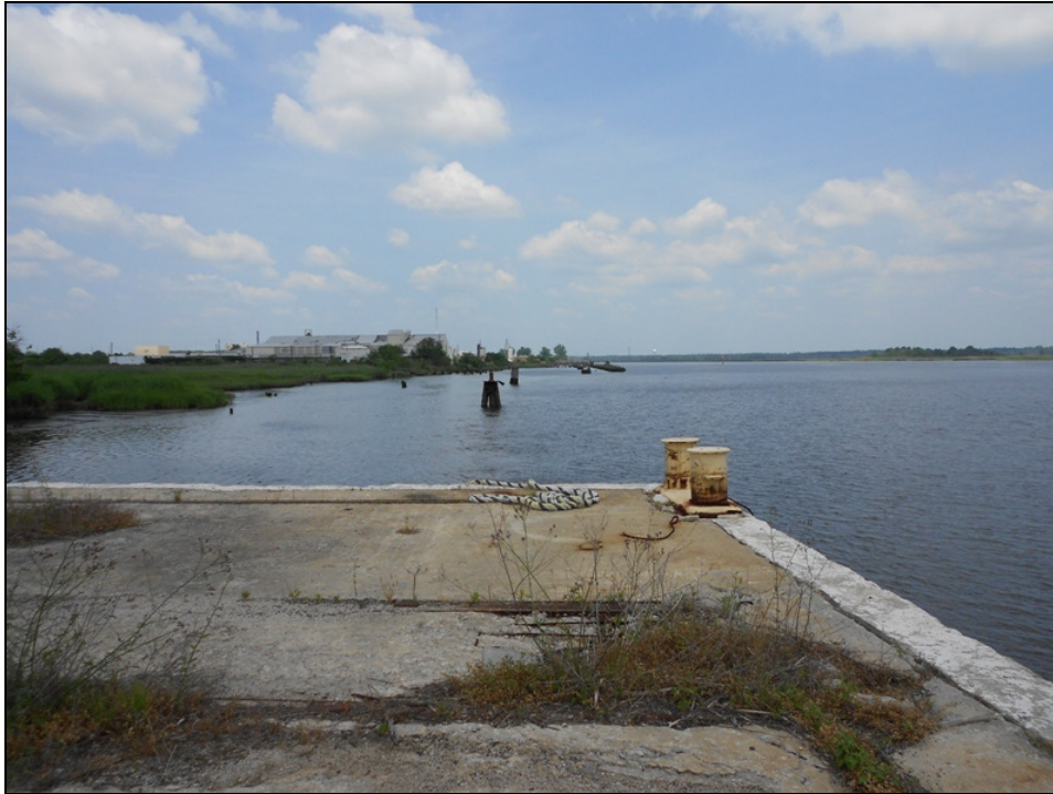
Photo 5. Horton Iron & Metal NPL site visit June 2011. View looking north along NE Cape Fear River from eastern end of source area toward northern most boat slip. Source: NC DPH HACE, June 2011.
