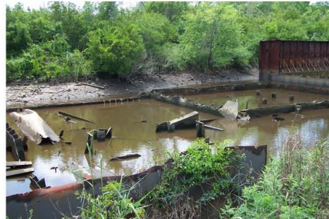
Remnants of ship breaking salvage operations (2011)
